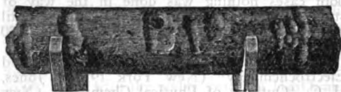
Electrolytically Pitted Water Pipe.
